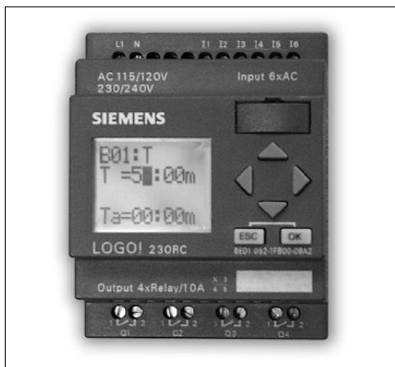
Siemens Logo Unit, located in MVP Panel
